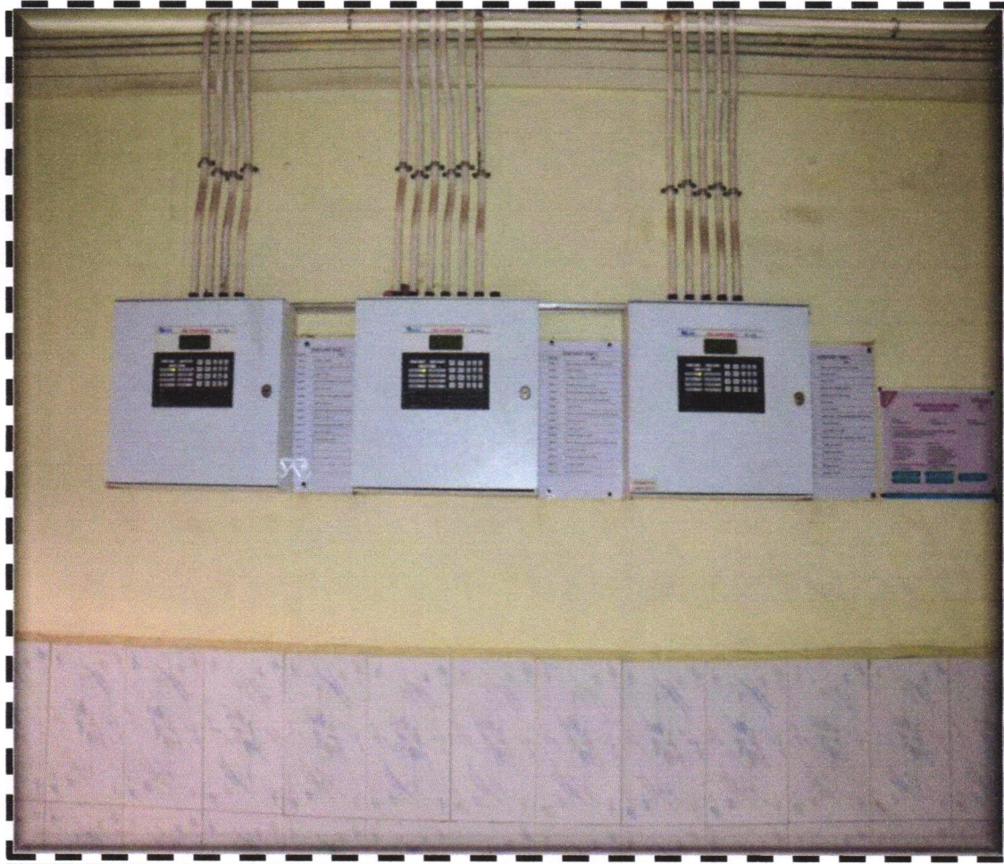
FIRE ALARM CONTROL PANEL – CHAVARA BLOCK
