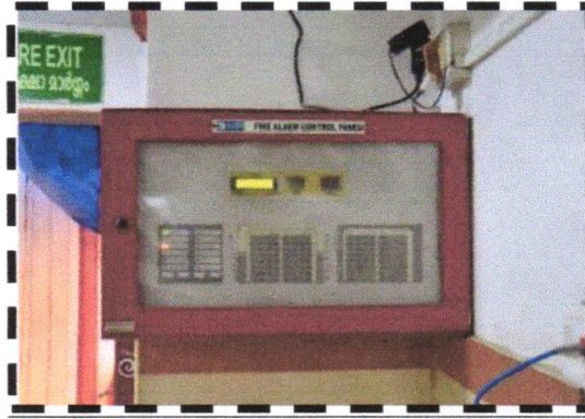
FIRE ALARM CONTROL PANEL – SACRED HEART BLOCK
