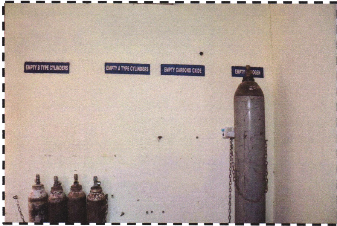
SEGREGATION OF CYLINDERS AT CHAVARA BLOCK
