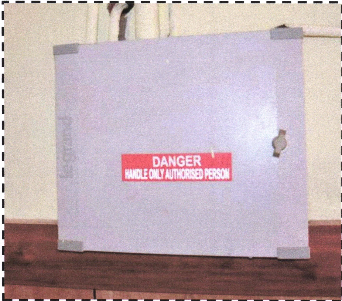
CHAVARA BLOCK- DISTRIBUTION BOX SAFETY MARKING
