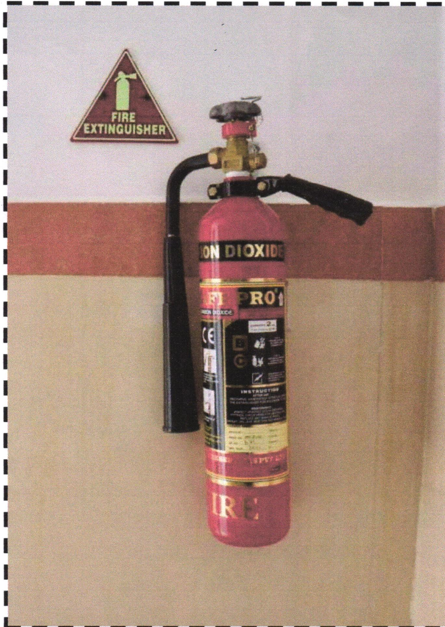
FIRE EXTINGUISHER – SACRED HEART BLOCK
