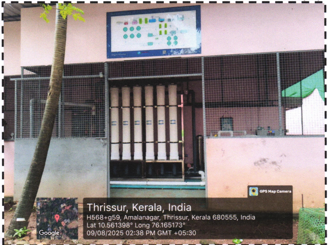
WASTE WATER TREATMENT PLANT
